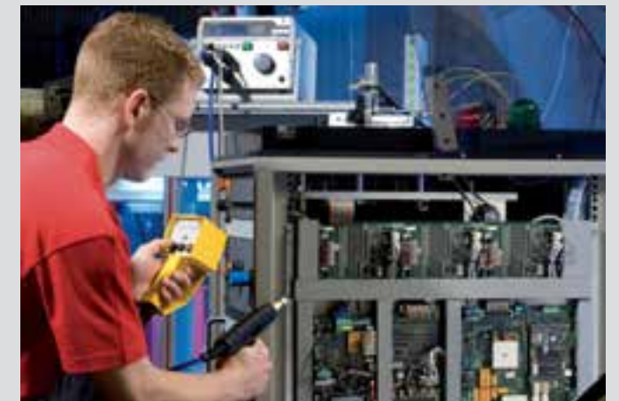
EN60204 test at a service cabinet
