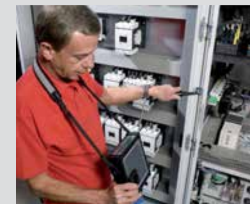
EN60204 test at a service cabinet
